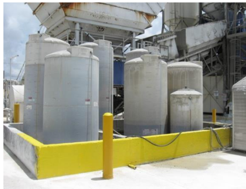
Plastic Admix Tanks in Containment
