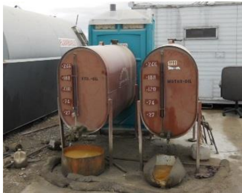
Steel Oil ASTs not in Containment
