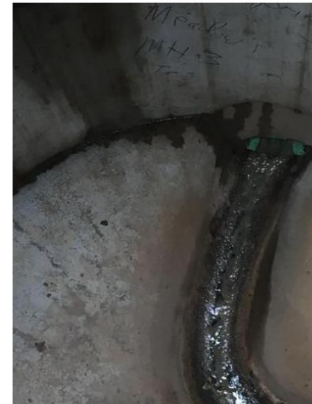
Manhole MS3 infiltration photo.
